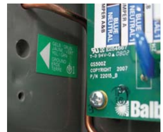
Ground in System Enclosure
