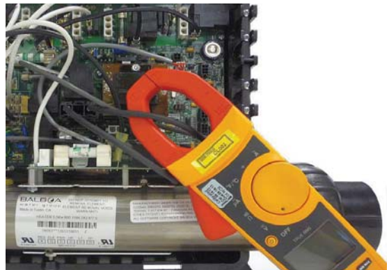
WHEN TESTING AMPERAGE
