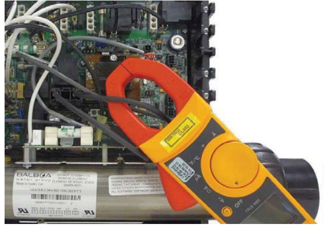
AMPERAGE HEATER TEST BP2000G1
